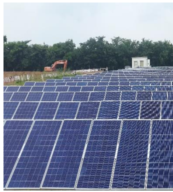
Phase 1 : 3.2 MW TKM Roof Top & Ground Mounted
